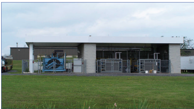
CATA's natural gas compressors.
